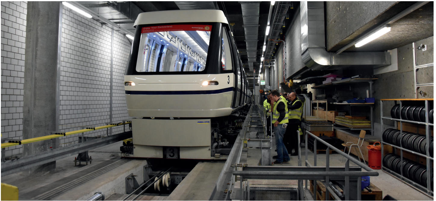
An empty Skymetro train arrives at the end of the Terminal E turnback track. The white pulleys are about to lower the right-hand cable and raise the left-hand cable so the train can grip it and depart in the other direction. Both cable sections are part of the turnback's cable loop.
