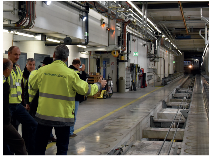
Beat Dübendorfer shows us the Skymetro workshop as a train enters the Terminal E crossover. A separate cable loop pulls trains into the workshop. The circles show the placement of each car's 28 air pads.
