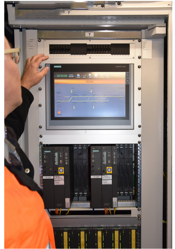
Chigny's Maintenance Terminal.
