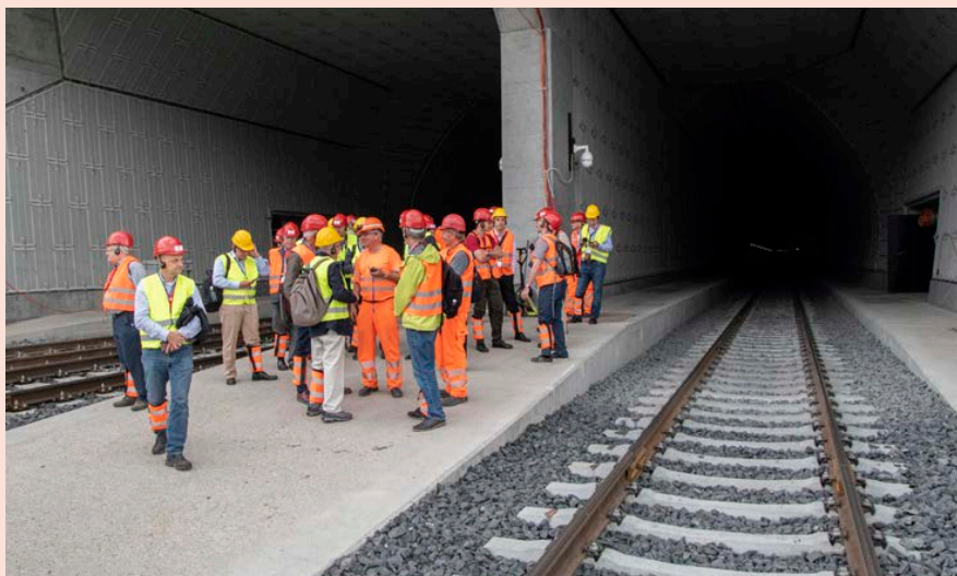
Members reflect on their 1-km walk through two tubes of the Ceneri Base Tunnel.
